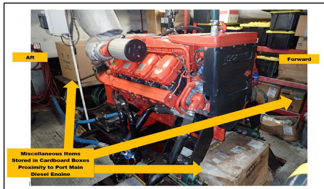
Figure 4: Combustible materials stored in the engine room.
